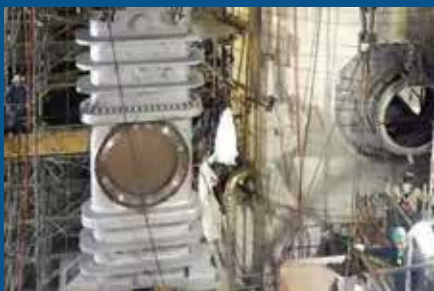
FCC Reactor Isolation
